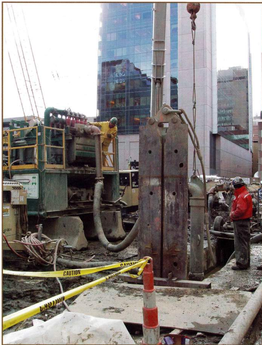
East Coast Slurry operates a Derrick de-sanding machine during construction of slurry wall at new Center for Life Science tower in Boston.
