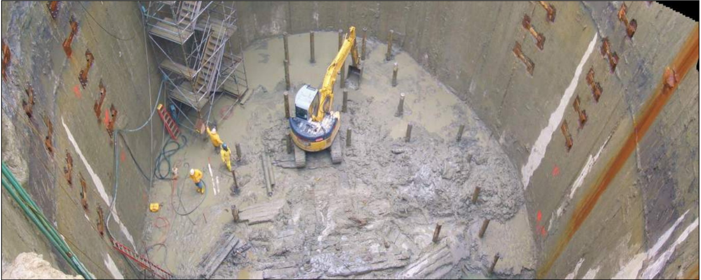
Unbraced Slurry Wall Earth Support System For Future 60' Deep Pump Station. Minipiles Will Provide Foundation Support for the CIP Pump Station.
