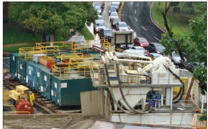
Sotress Desanding Plant
