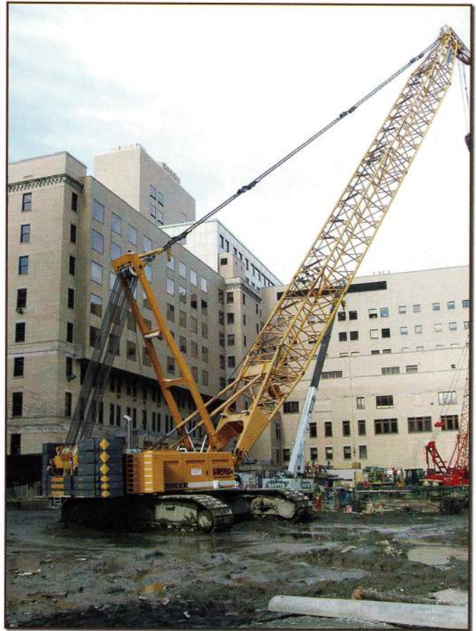
HUB Foundation's Liebherr is principal crane for lowering giant rebar cages into trench.
