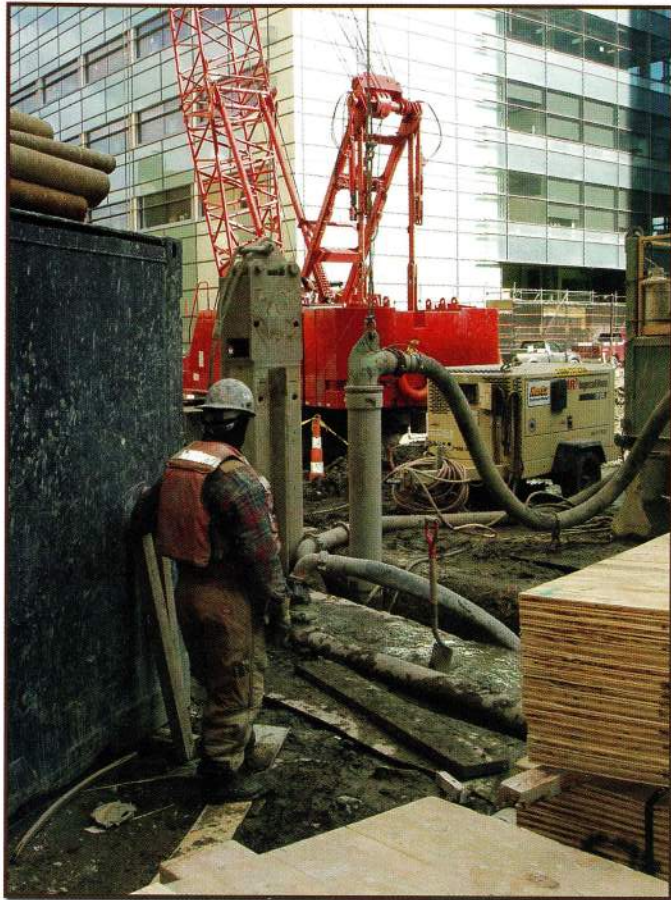
With Manitowoc 666 excavator in background, worker observes operation of air-lift pipe for recycling slurry from 100-foot-deep trench.
